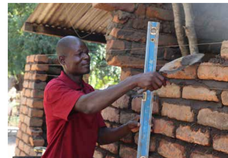
April Sipiliyano repairing his house in the aftermath of a devastating cyclone
